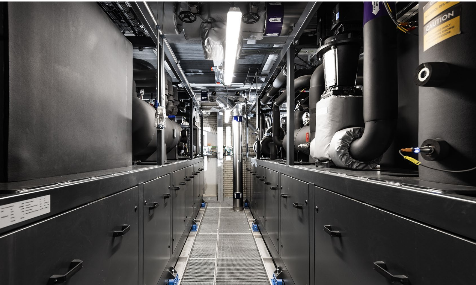
The three CO 2 heat pumps from Fenagy provide 5.2MW of heating capacity and 3.6MW of cooling capacity. Photo credit: Fenagy
