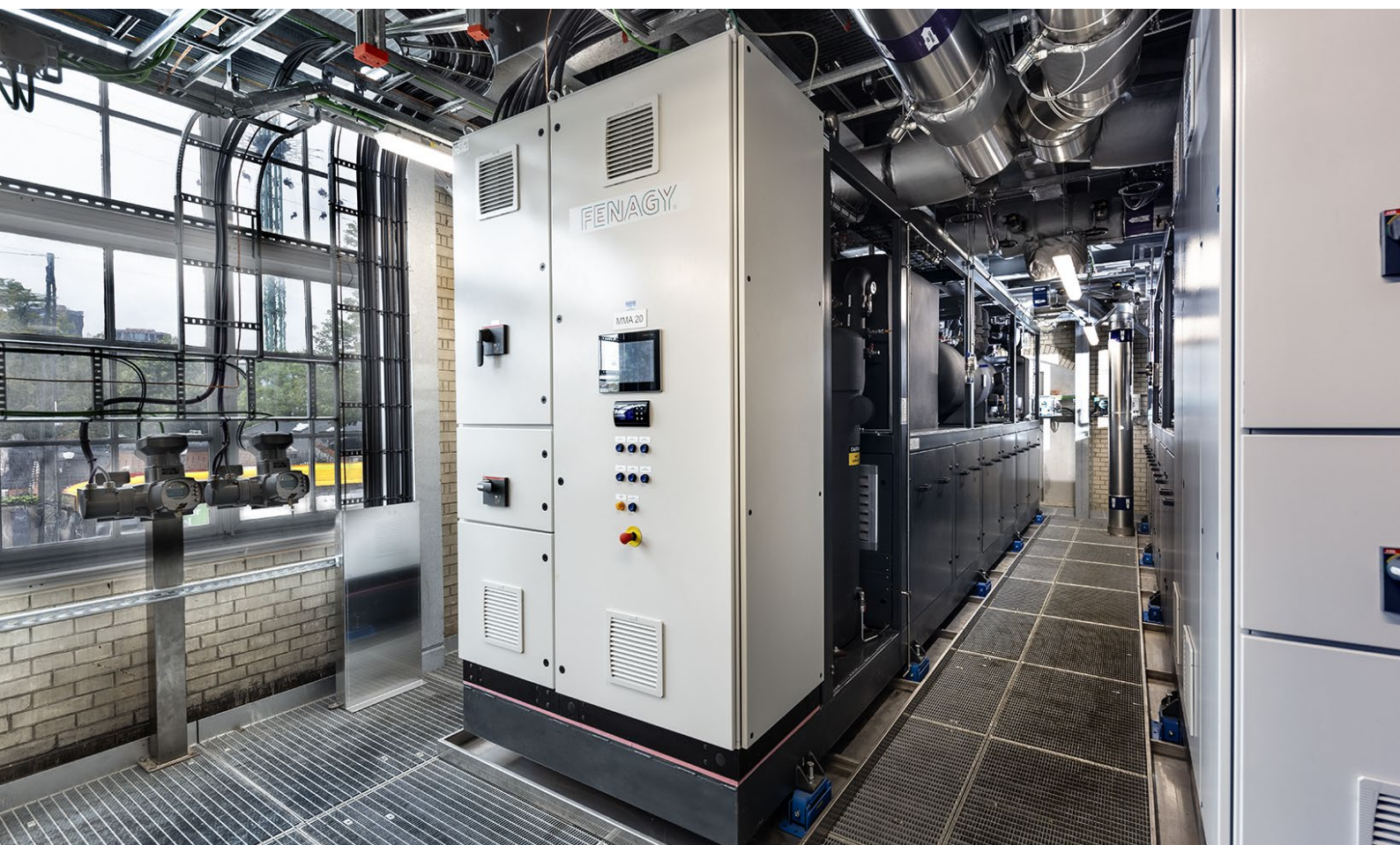
Two of the three Fenagy CO 2 heat pumps installed at the Tietgensgade facility with compressor panels and vibration feet. Photo credit: Fenagy
