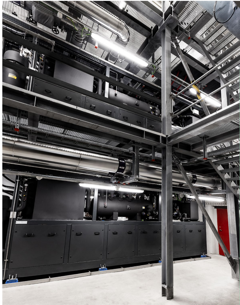
To get around space constraints, a mezzanine level was installed so the heat pumps could be stacked on top of each other. Photo credit: Fenagy
