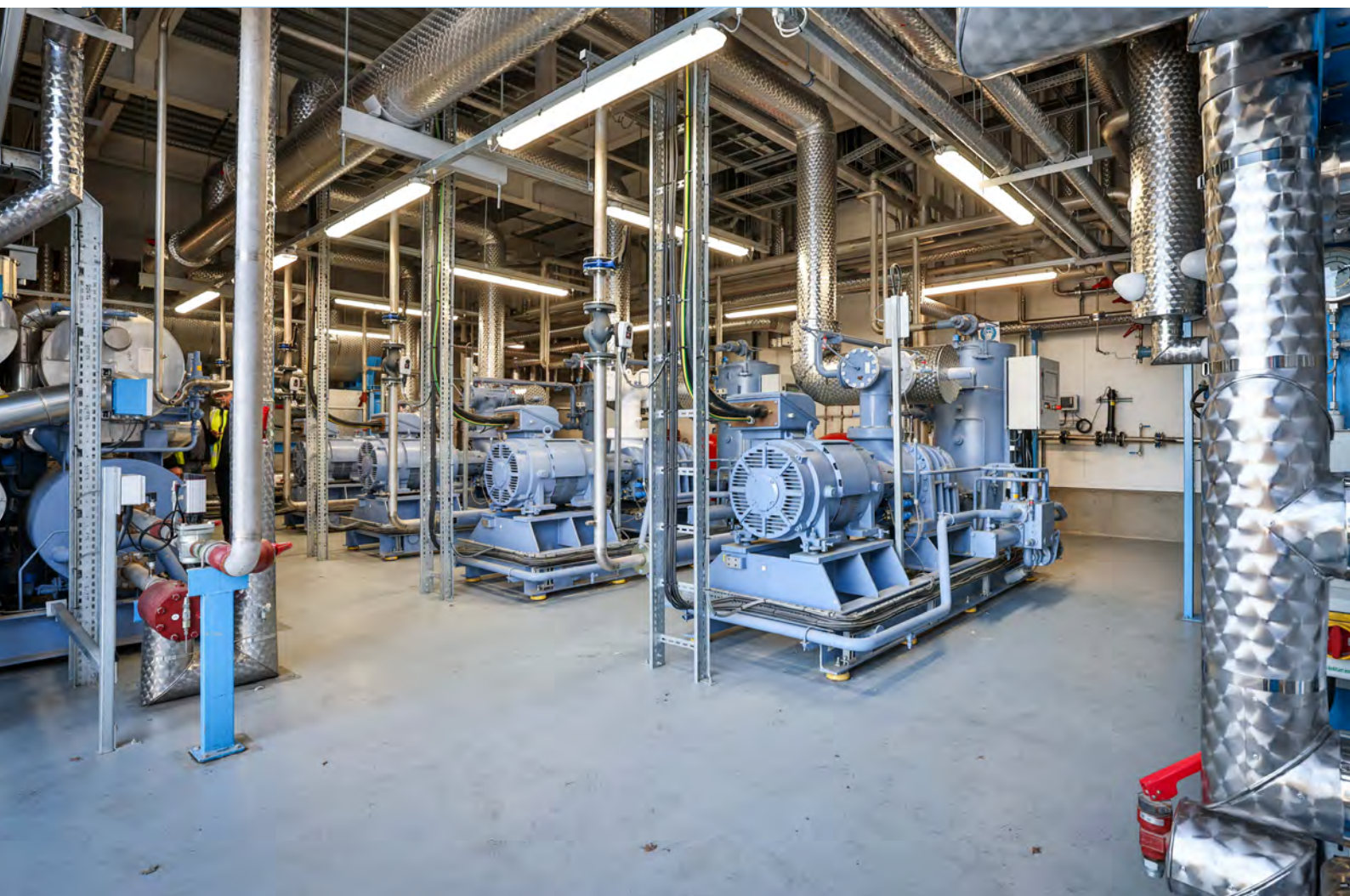
Engine room at Cranswick's prepared poultry facility in Hull, U.K., with four GEA screw compressors (right) and heat pump (left).
