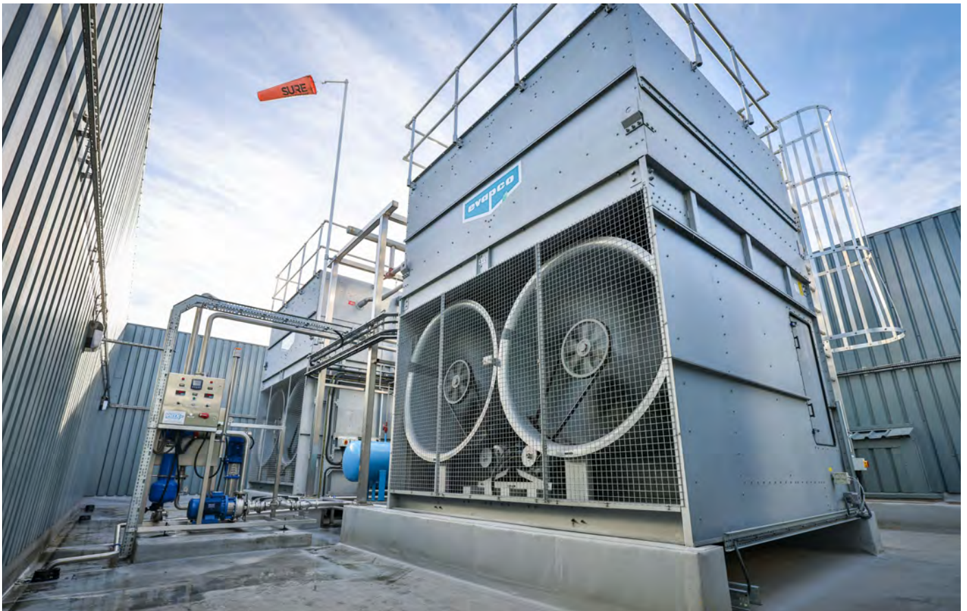
Evapco evaporative condensers on roof of Cranswick's prepared poultry facility, with ammonia receiver (light blue) and chemical-free water treatment system.
