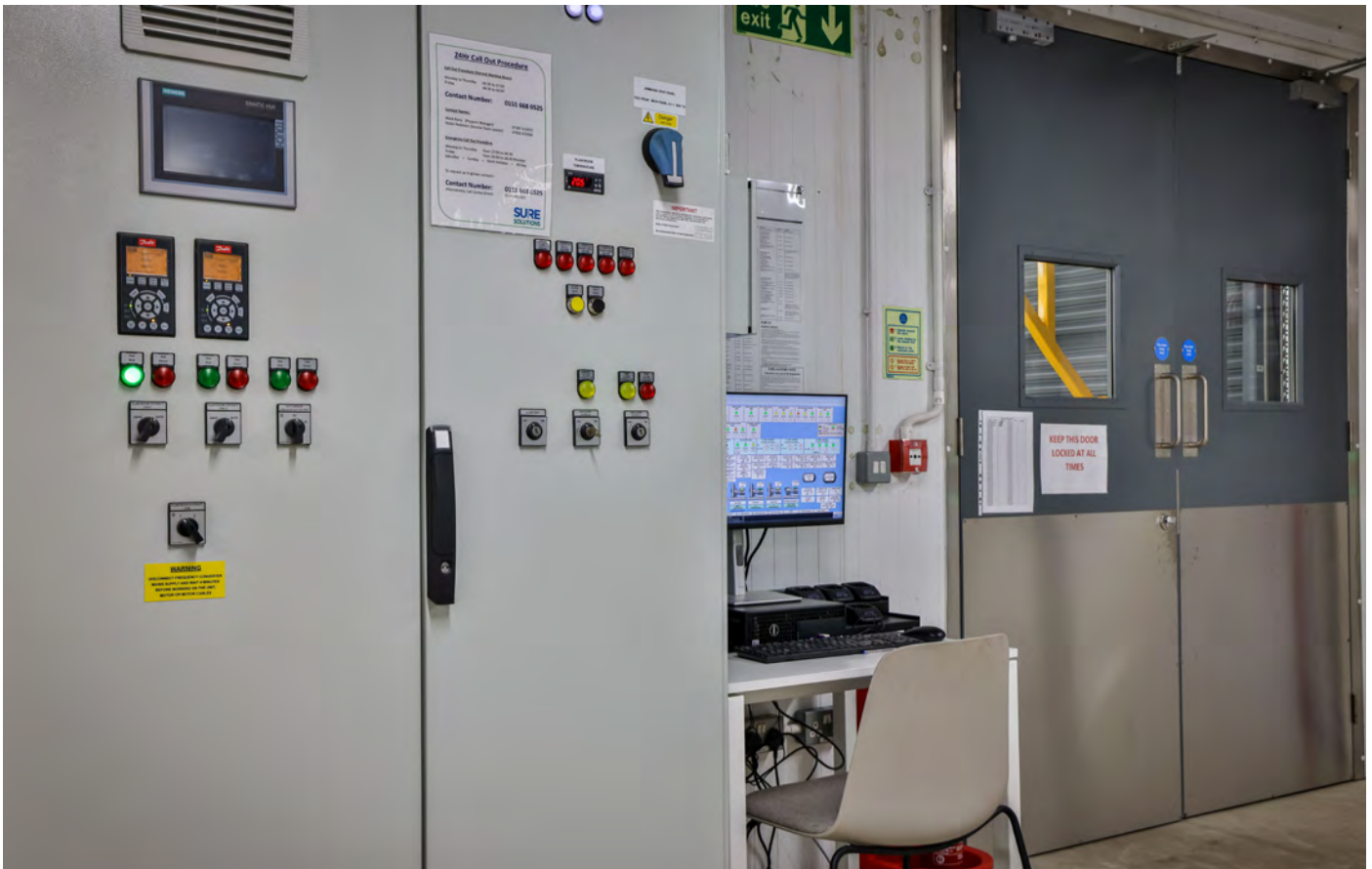
Computer (right) at Cranswick's prepared poultry facility that manages all switchgear, variable speed drives, leak detection panels, ventilation panels and other components, with ammonia leak-detection panel (middle) and ventilation panel (left).
